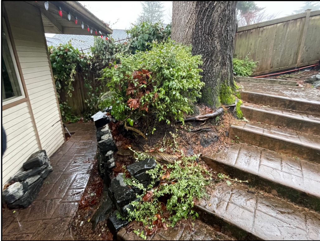
Photograph 4. Limited rooting area at the base of tree 170 causing uplift of the adjacent steps and damage to the existing retaining wall.
